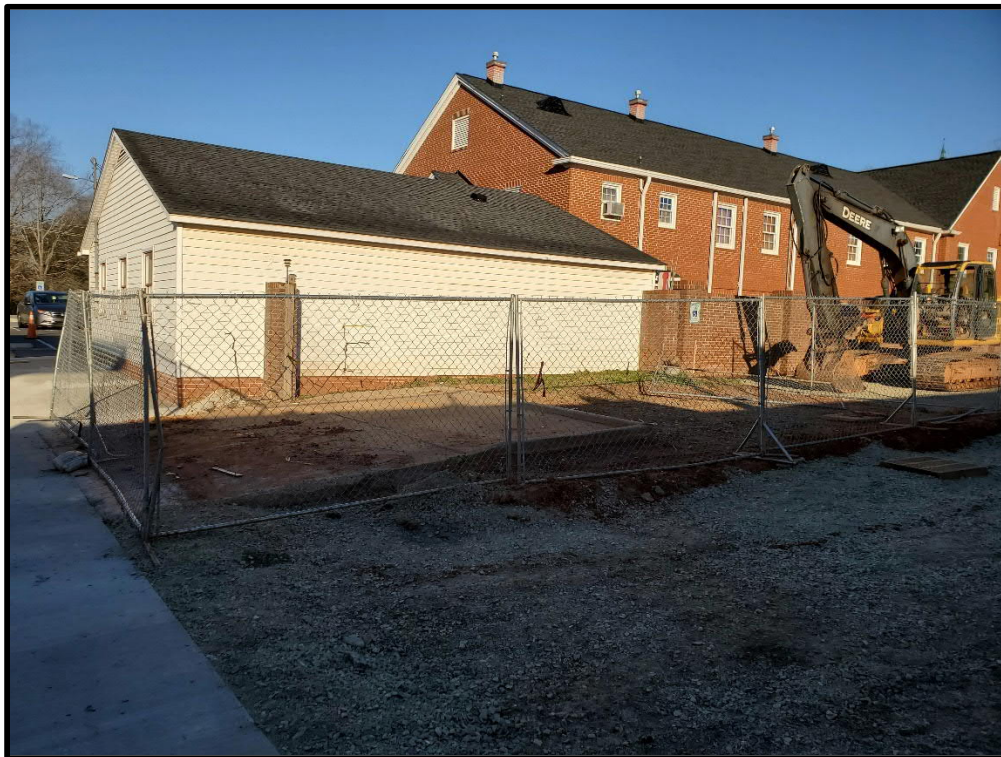
Figure 5. Overview of Stedman Cemetery (inside fencing) Prior to Concrete Removal, View Northwest.
